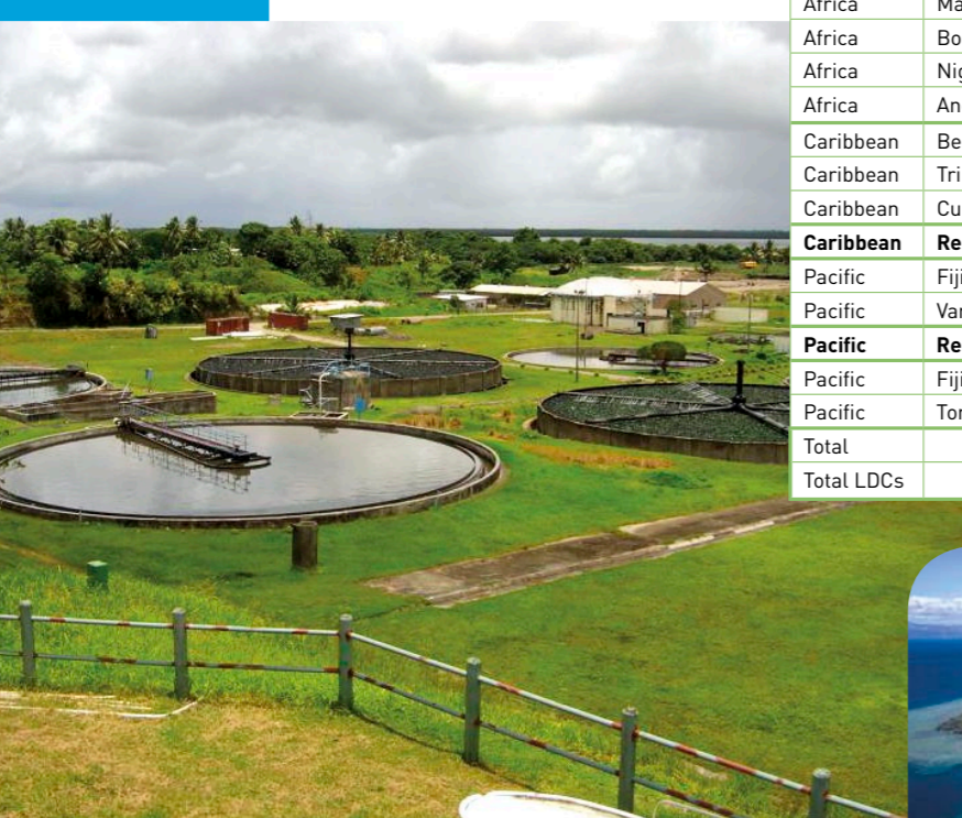
Kinoya Sewerage Treatment Plant in Fiji where Biogas Capture and Flaring is being implemented
