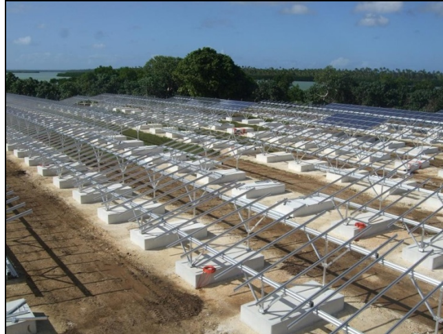
Figure 4 View of solar farm
