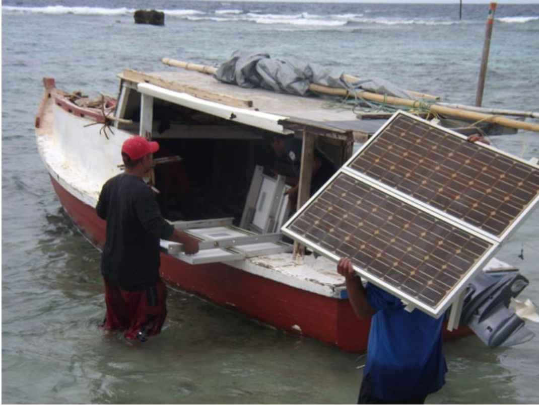
Photo: Ha'apai solar home system installation, EESLI project in 2009. Curtsey to Tonga Energy Planning Unit.
